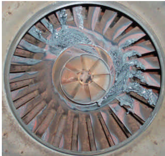
Figure C.3 – Burner Damage Caused by Flashback
